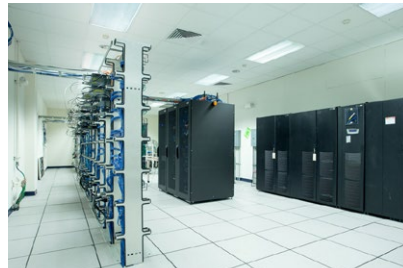
Server & Data Room
